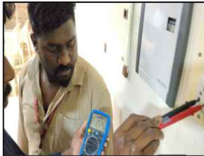
Voltage intensity measured at the Campus
