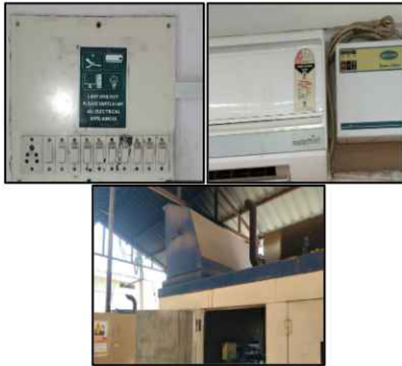
Energy conservation facilities observed in the Campus
