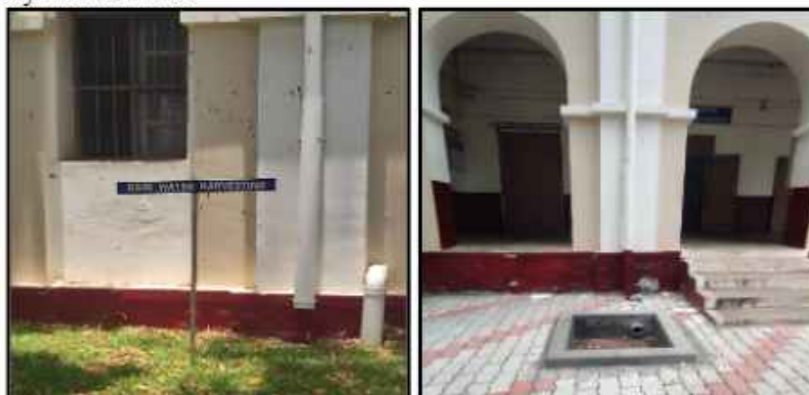
Rainwater harvesting system observed in the campus
