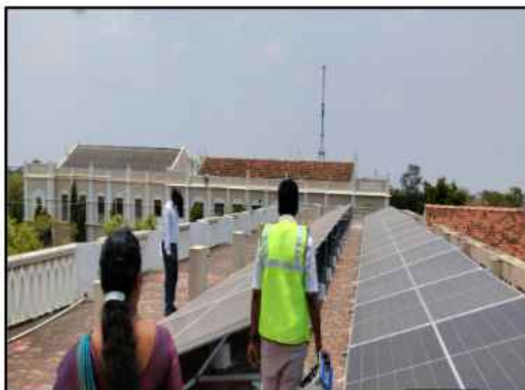
Solar panel observed in the campus
