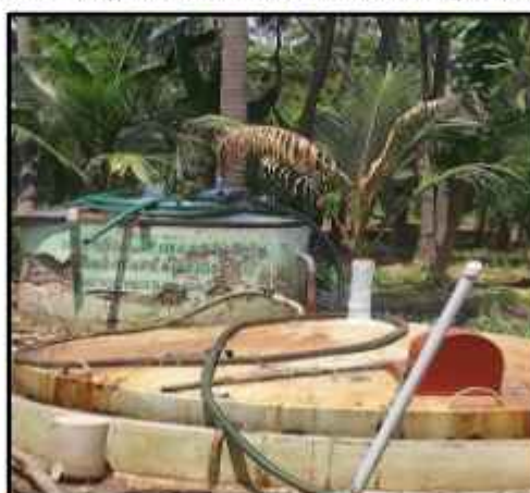
Biogas Plant is available in the campus
