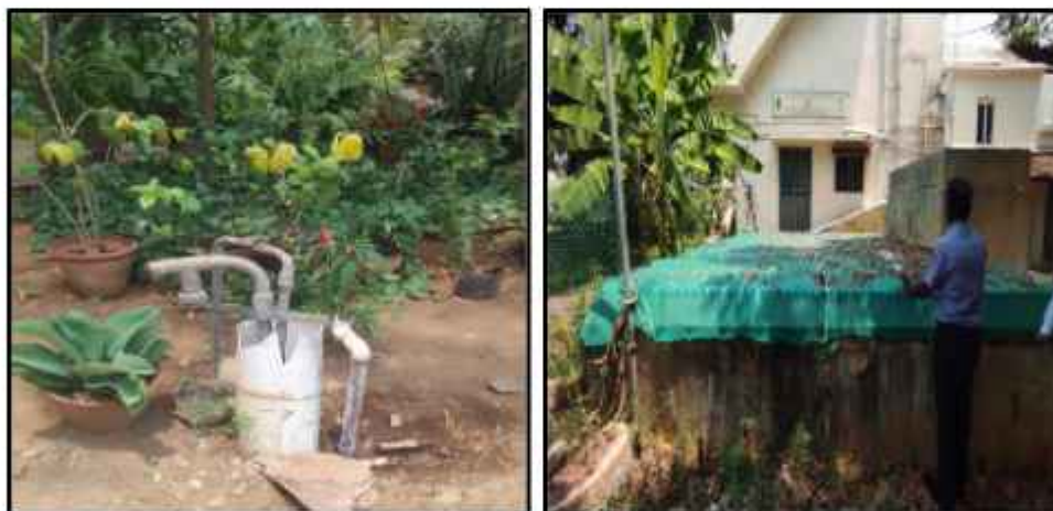
Bore well observed in the campus
